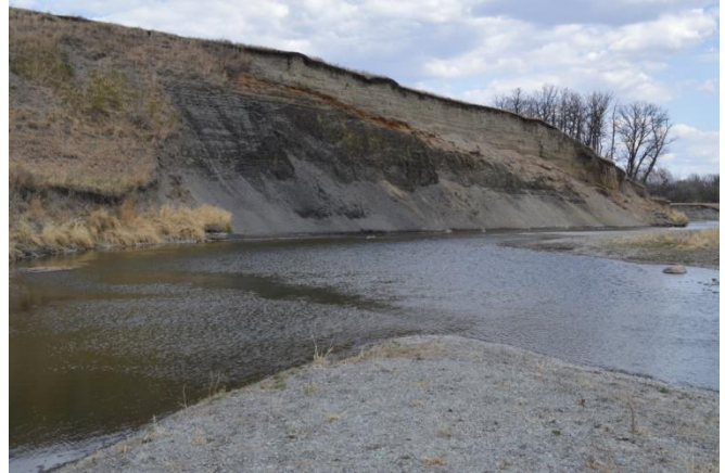
View of a bank along the Pembina River.
